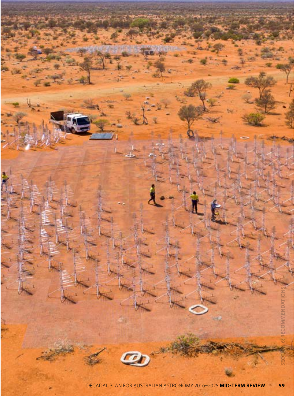
An aerial view of the construction of the Aperture Array Verification System (AAVS) station, a testbed for Square Kilometre Array technology. CREDIT: ICRAR/CURTIN
