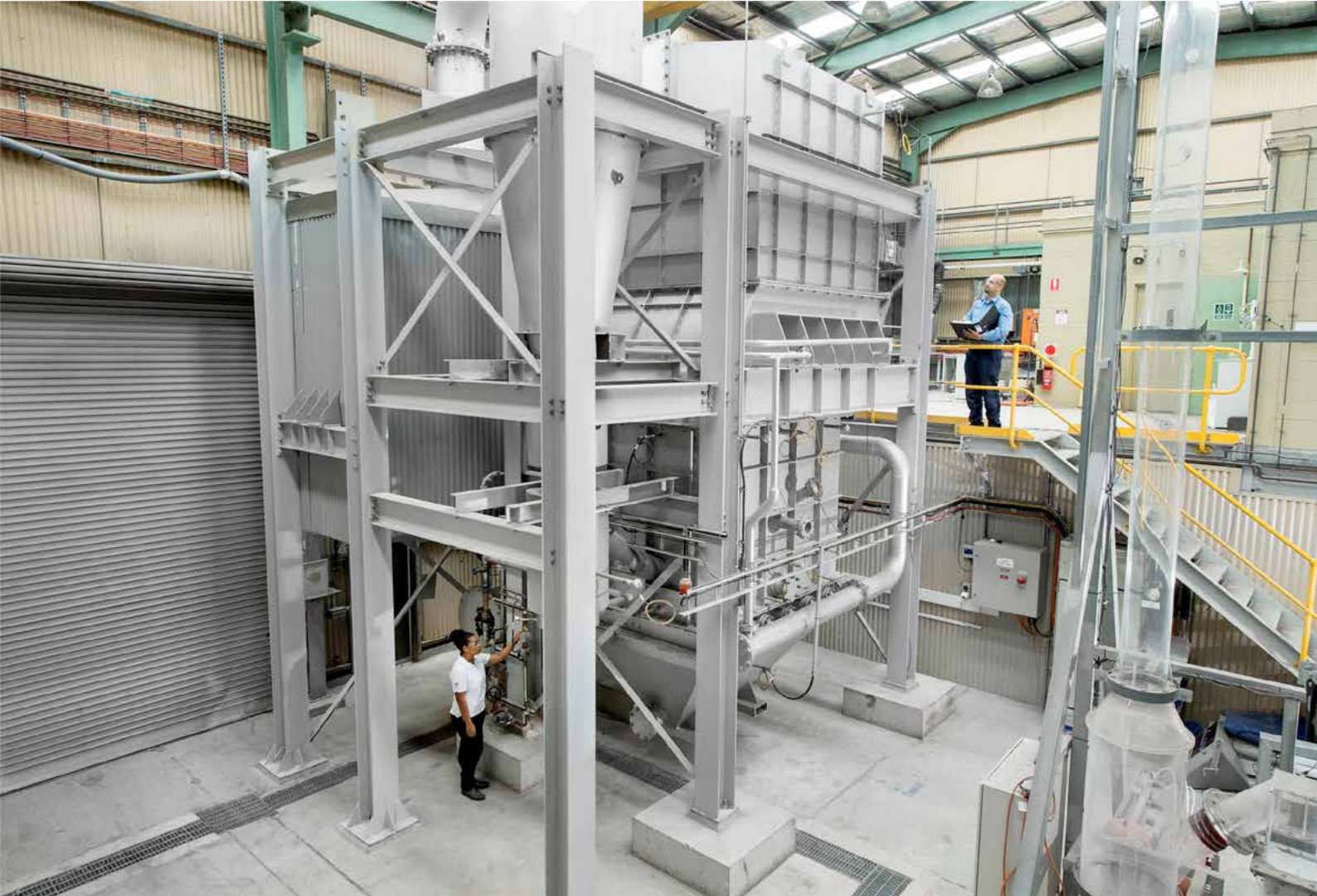
A picture of the VAMCO chemical-looping technology developed by Laureate Professor Behdad Moghtaderi and his team at the University of Newcastle for capture of CO 2 or methane.
