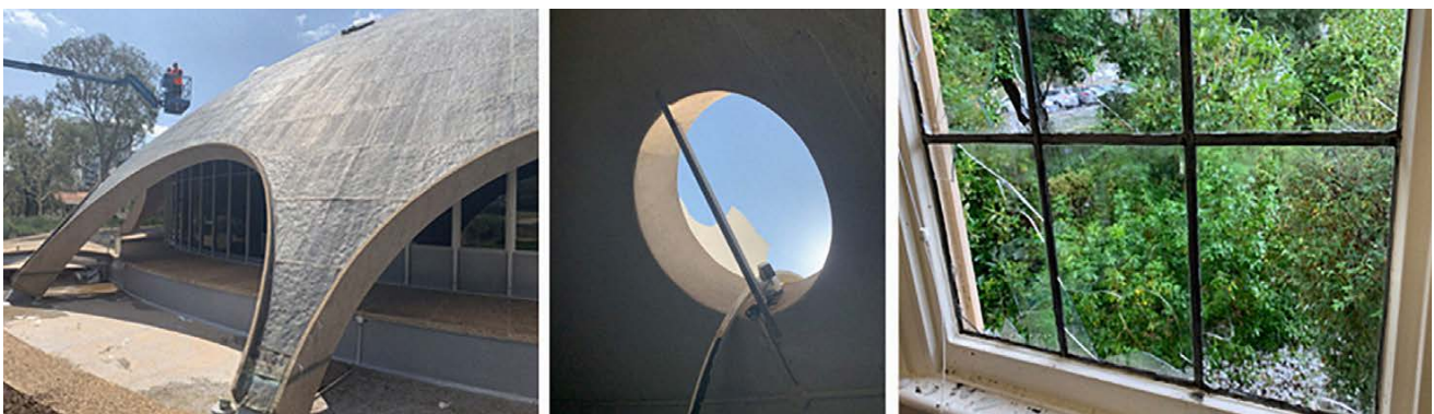
(from left) Large hail caused pitting on the copper roof of the Shine Dome; a broken skylight in the Shine Dome; and one of many broken windows in Ian Potter House.
